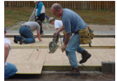
John Sizer of Silicon Logic Engineering helps to build a two car garage.
